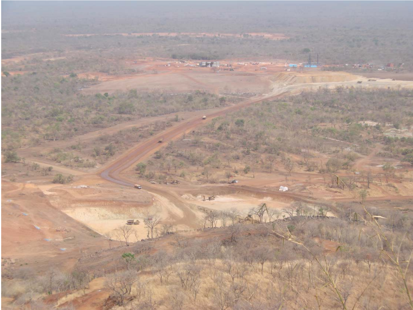
Attachment 3 – Waste being stripped from the Sabodala pit to ready the ROM for ore storage in Q3
