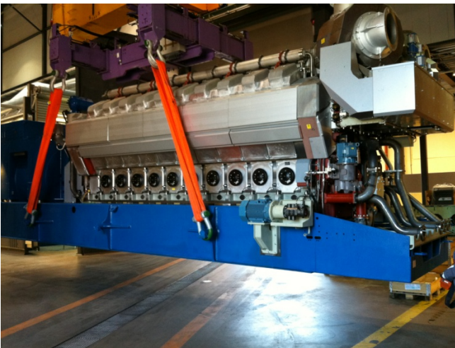
One of the power station engines being completed in Finland
