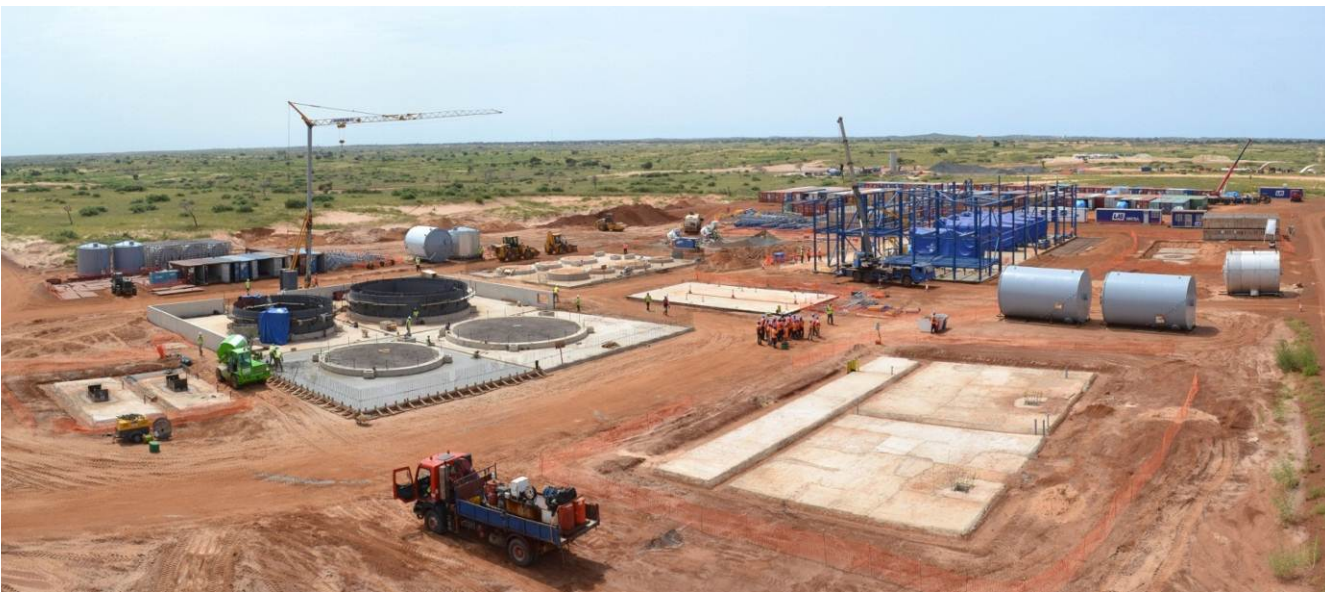
Power station engines are positioned on foundations while erection of structural steel for engine hall commences
