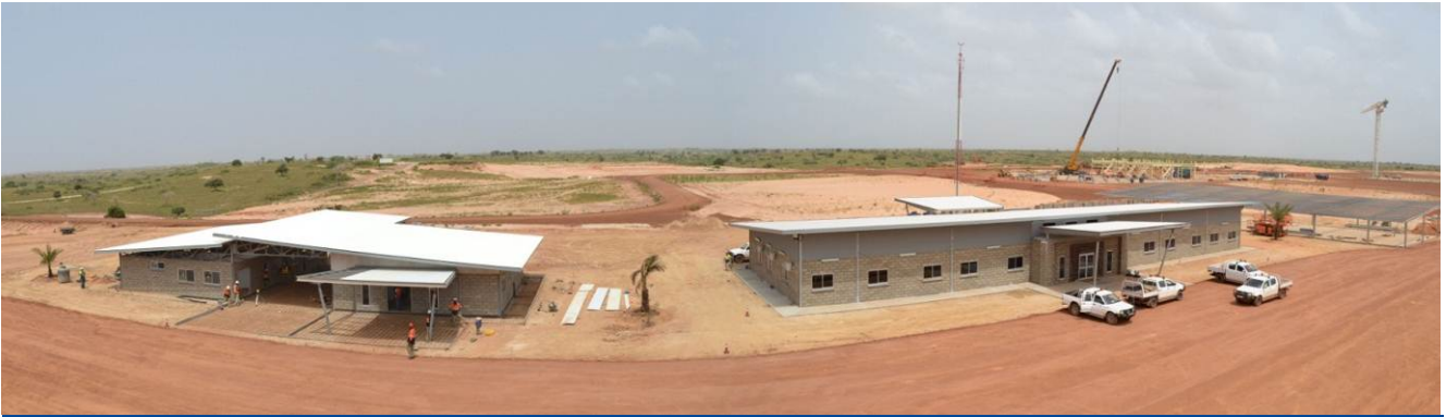
(Left) New ERT and clinic building nears completion. (Right) Administration building now complete at MSP
